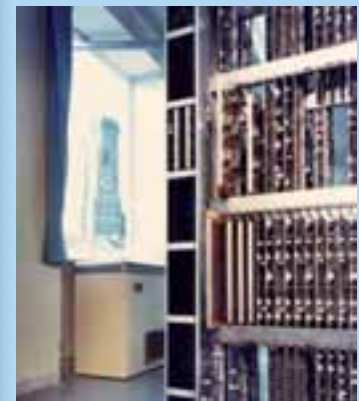
Erstes elektronisch gesteuertes Fernsprechart Deutschlands in München 1962. Germany's first electronically controlled telephone exchange is commissioned in Munich in 1962.
